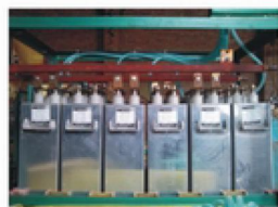
20吨感应炉配套电容柜 capacitor cabinet for 20 tons induction furnace
